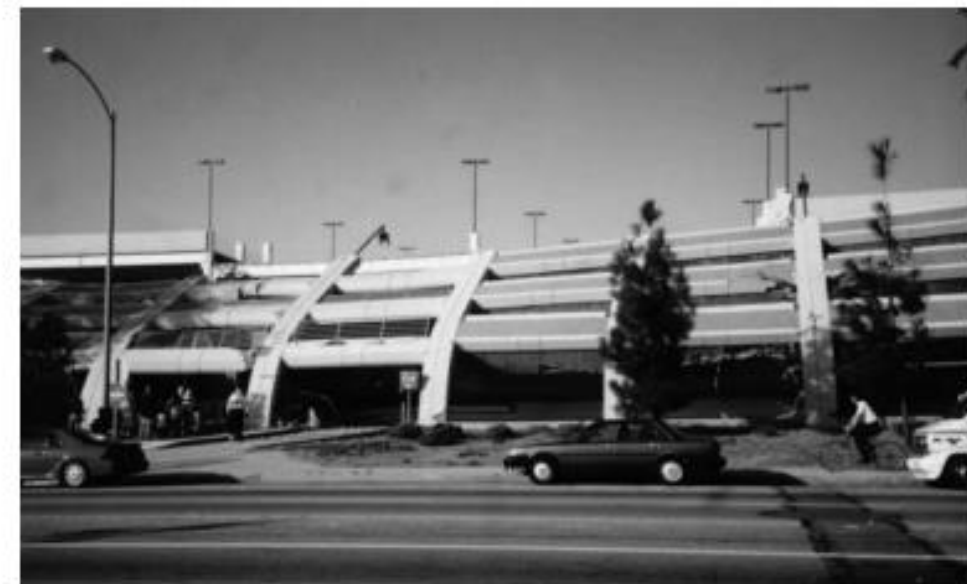
Figure 3 California State University Northridge parking structure built in the early 1990s collapsed after the 6.7 magnitude 1994 Northridge earthquake.
