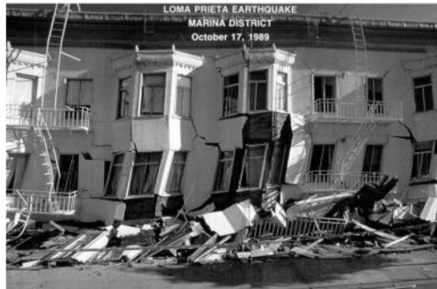
Figure 2 Marina District Apartment building damage during the 6.9 magnitude 1989 Loma Prieta earthquake. Two nearby public schools were not damaged and were used as emergency shelters.
