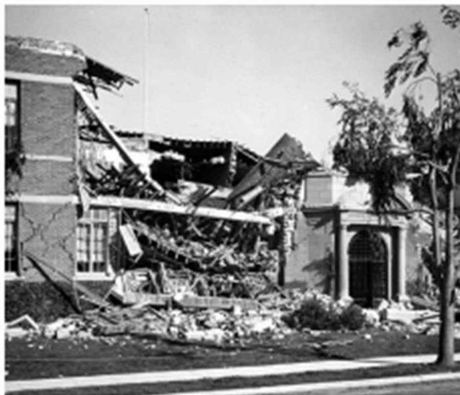
Jefferson Junior High School, The Field Act & Public School Construction: A 2007 Perspective
